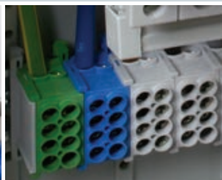
The terminals permit connection between the different supply lines.
