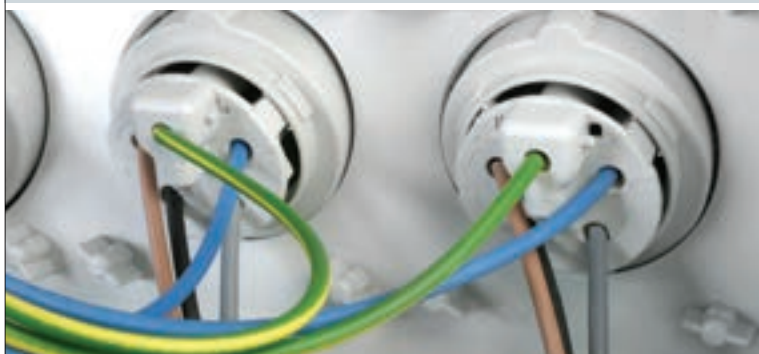
Ample space for wiring the bases, performed according to the REBT.
